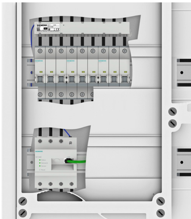
7KT PAC1200 multichannel current measuring system installed
