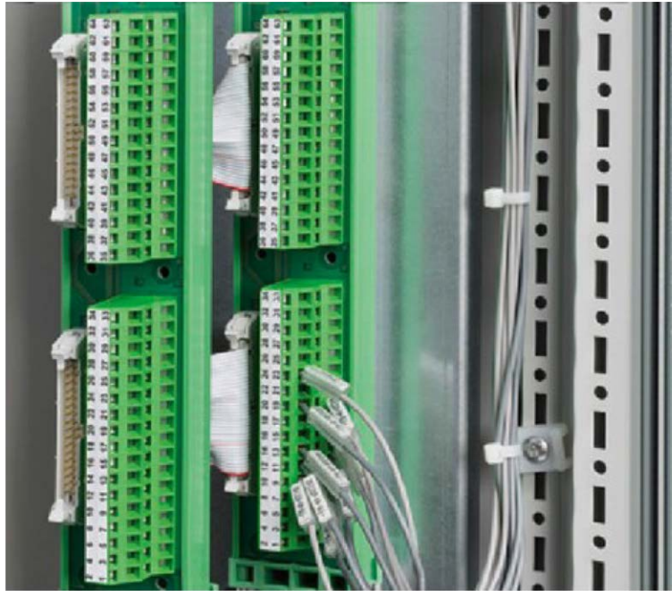
Figure 10-92 Terminal Module Cabinet
