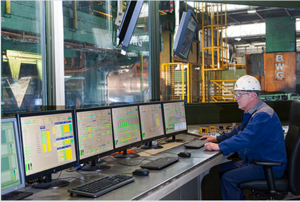
Reference: V7 Control room
