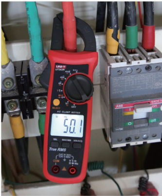
High voltage (600V) frequency measurement
