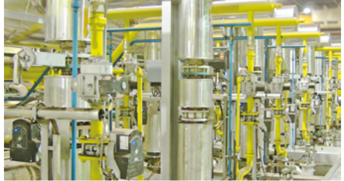
Walking beam furnace with overhead firing
