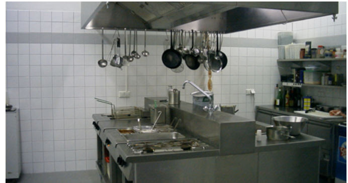
Filter monitoring in kitchens
