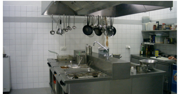
Filter monitoring in kitchens
